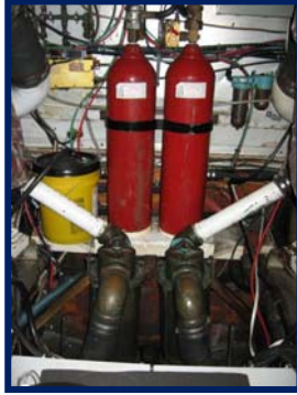
Engine Room Fire System
