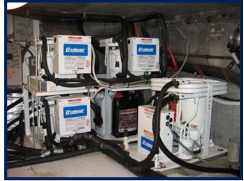
New Air Compressor System
